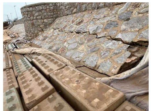
Temporary defences were installed in 2023 to prevent further deterioration of Exmouth Sea Wall. Image: EDDC
